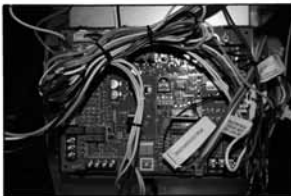
INTEGRATED FURNACE CONTROL
